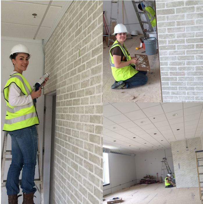
Natalie McKeever Goldman and Nicole McKeever helping to put some finishing touches on the walls.
